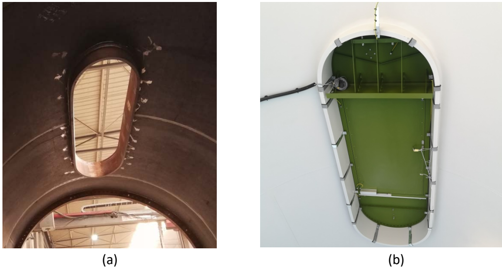
Figure 1. Photos of typical man-door openings (a) during fabrication (b) in the finished state
