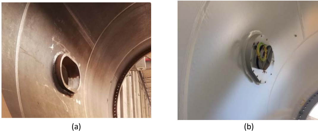
Figure 2. Photos of typical ventilation openings (a) during fabrication (b) in the finished state
